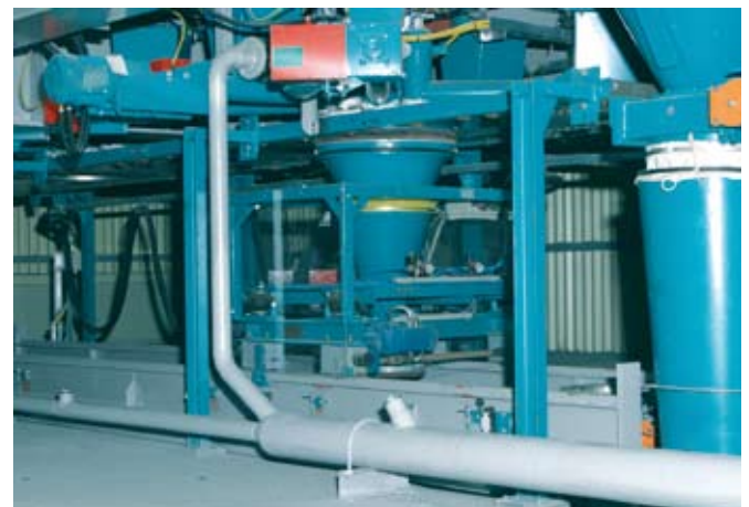
Fig. 5.3: Traversaler weigher in the mixing plant at Haniel Cement
