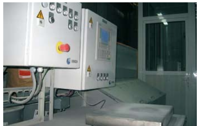
Fig. 3.5: Table scales and operator terminal for manual batching of additives
