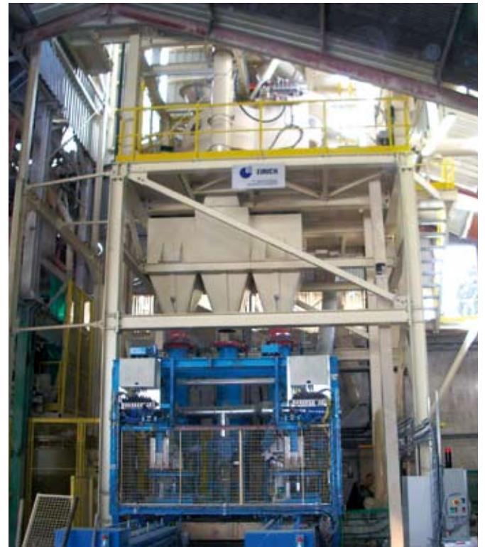
Fig. 7.2: Newly installed RV19 intensive mixer from Eirich
